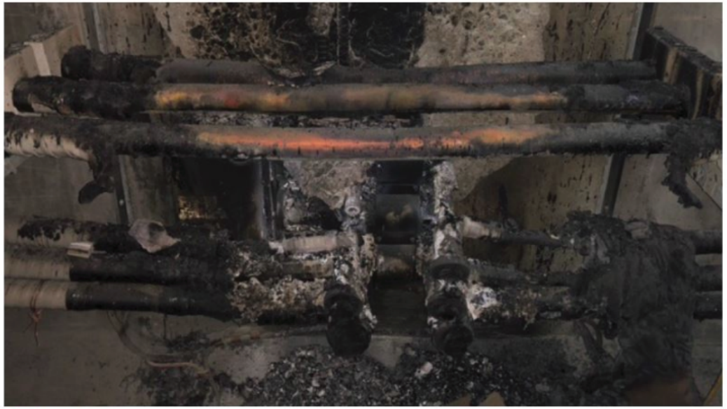
Photo from FOX 5 News showing the damage on the electrical equipment.
